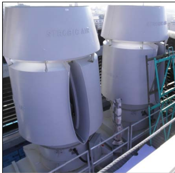
Figure 3 Laboratory Exhaust Fans
